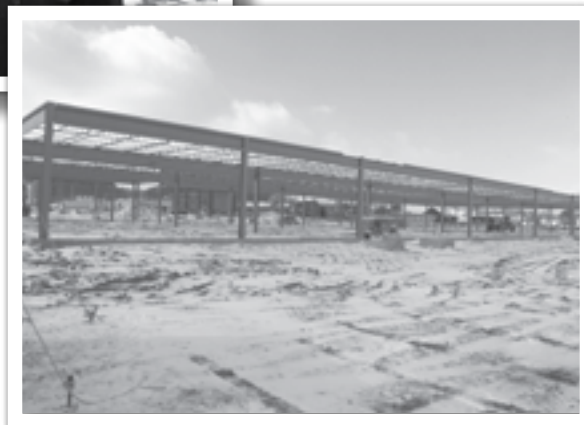
Initial work on the facility's structure is underway. Mercy plans to open its health center later this fall.
